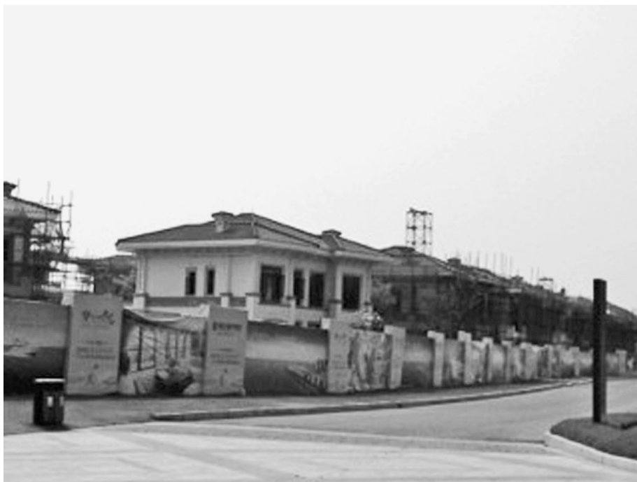
A luxury housing development in Hainan still selling at the top of the market but apparently abandoned. Photo by the author.
